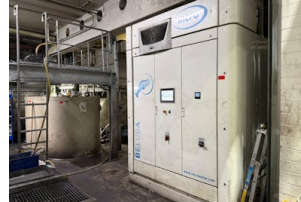
Evaporator system Incro, Beluga Year of manuf.: 2021
